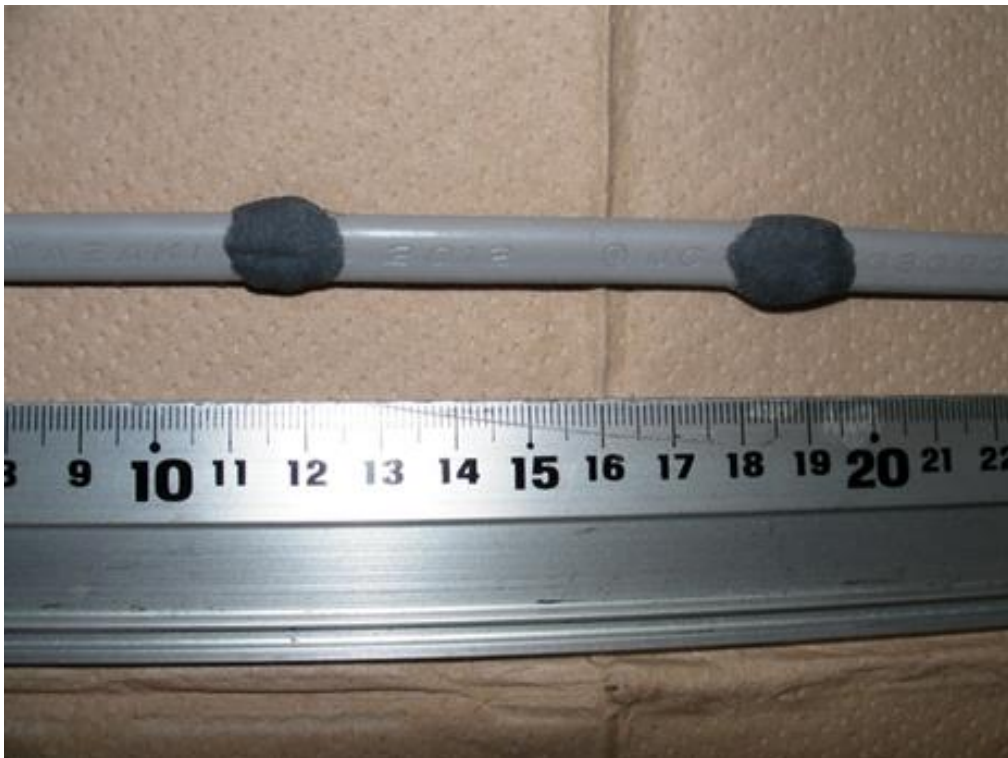
(b) To ensure no movement of the conductors, fire resistant putty is used
